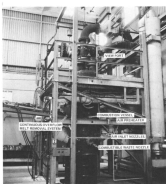
Figure 4. Santa Susana molten salt test facility
