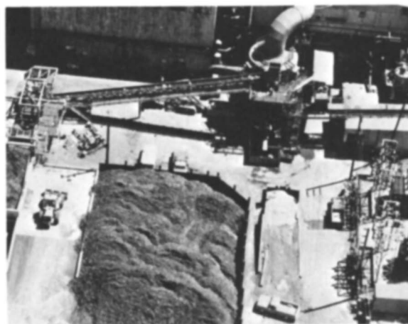
Figure 3. View and schematic of FBC boiler installation
