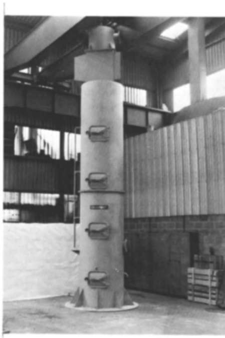
Figure 5. Gas scrubber with condenser mounted on top
